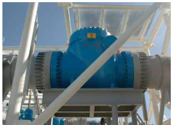
Taper-Lok® on 48 inch Subsea Check Valve
